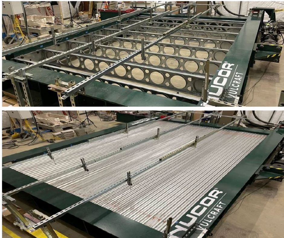
Figure 2: Photograph of the CFS diaphragm fixed in the rig before and after the steel deck installation
