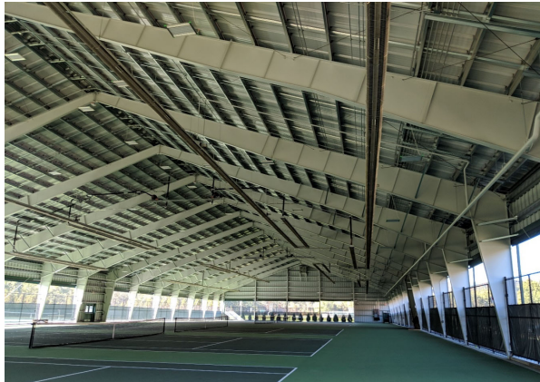
(a) Clear-span gabled portal frames with nonprismatic columns and roof girders (courtesy of Lee Shoemaker, MBMA)
