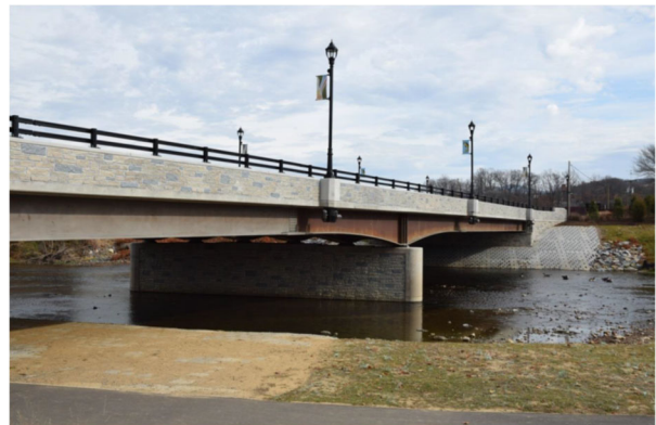
(d) Highway bridge with variable web-depth I-girders (courtesy of Jason Provines, VDOT)
