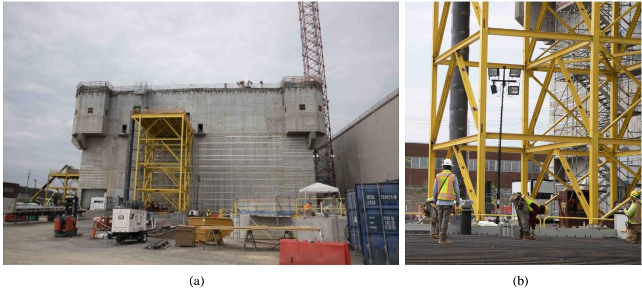
Figure 1.1: Typical 54 Foot Temporary Construction Work Platform (a) Overall View; (b) Close-up View of Chevron Bracing After Immediate Connectors Added
