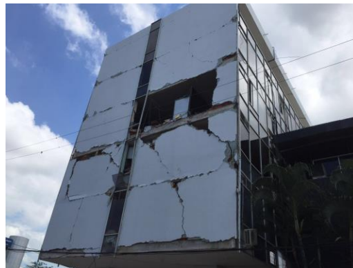
Figure 2: Cladding damage in a building after the 2016 Muisne Earthquake
