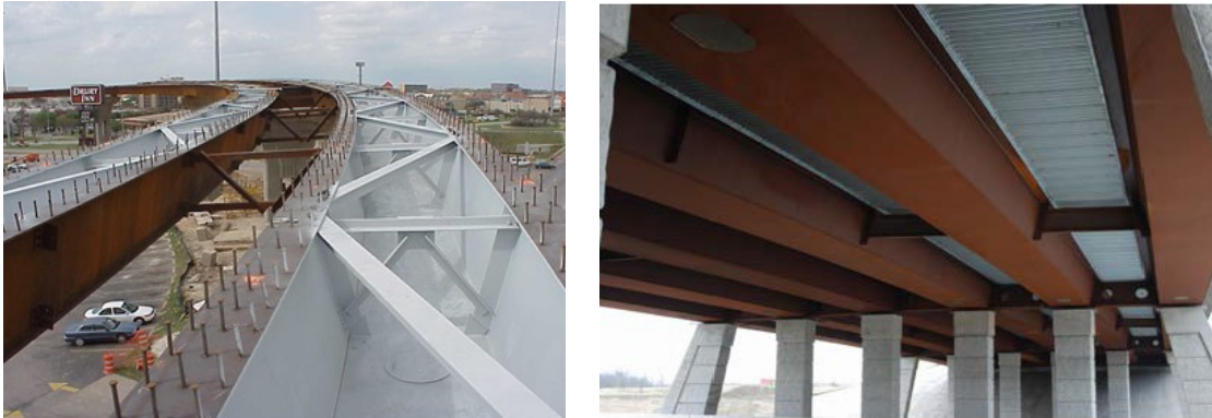
Figure 1 – a) Bracing Systems in Twin Tub Girder during Construction, b) Shallow Tub Girder System Waco-Texas
