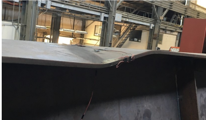
Figure 8 - Local Buckling of West Top Flange at Midspan - Offset Top Flange Girder
